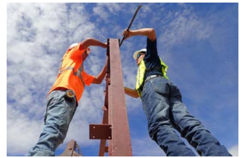
Welding and Construction Tech students helped build a storage shed for each program.
